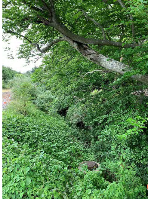
V6 - Steep bank between access track and woodland along Carrickmines Stream
